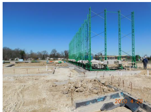
Masonry scaffold set and ready for masonry install on south wall of gym
