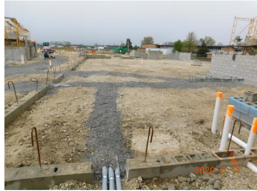
Gray stone showing paths of underground electric installation
