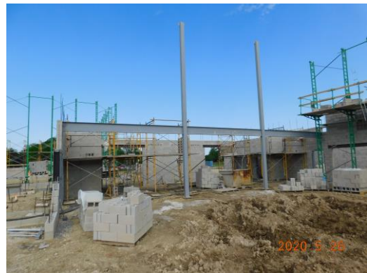
Steel column installation on the West end of the student dining area
