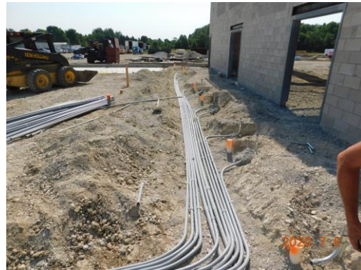
Underground electric installation in the kitchen
