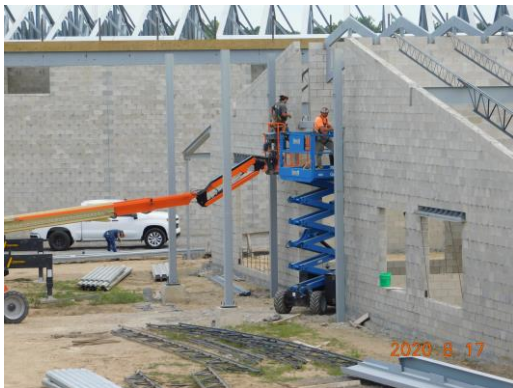
Steel installation is taking place at the main entrance for the canopy
