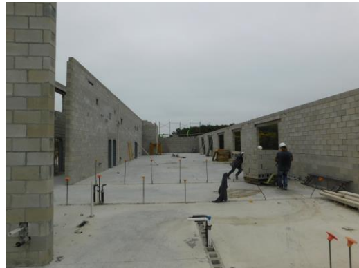
Unit D bearing walls at corridor and south wall are now at bearing height.
