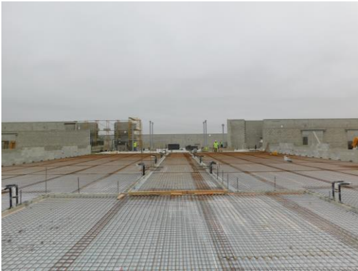
2 nd floor of Unit E being prepped for the concrete pour this week.
