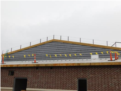
Insulation and Z furring installed on the east side of the gym roof for the metal panels
