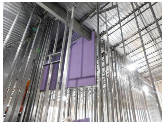
Drywall tops being installed in the admin area where roof is dried in
