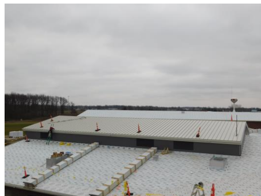
Metal roof panels installed on student dining and staged for kitchen area
