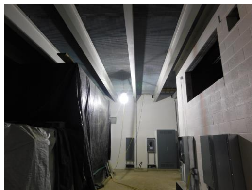
1 st floor mechanical room in Unit C has received block fill and ceiling paint
